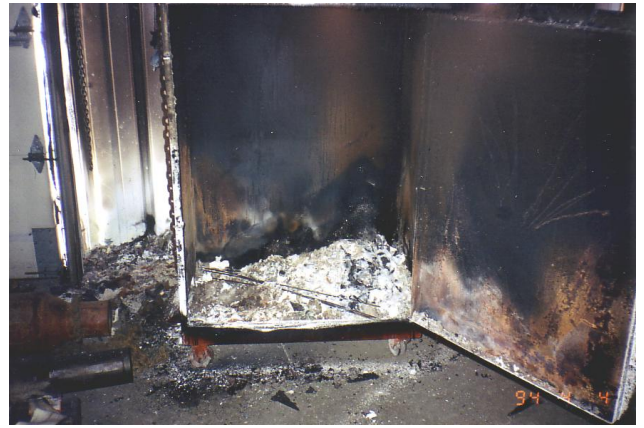
Shop magazine, note debris left from stored charges within the magazine.
